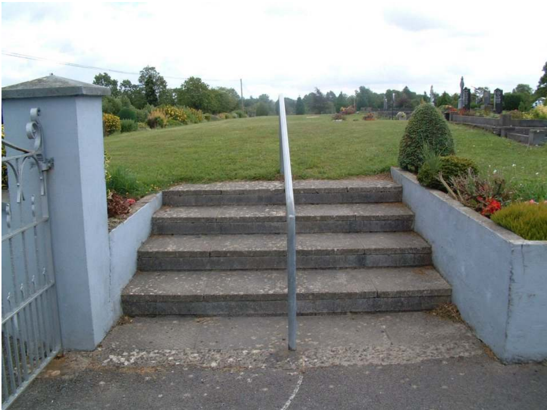
Handrail at 'Split-Level'
